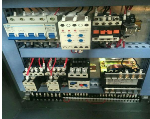
Control box electric
